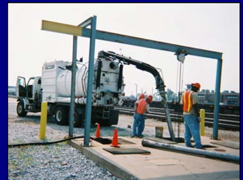
EWI field technicians perform oil / water separator cleaning using the company-owned Guzzler.
