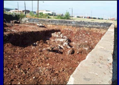
Excavation of 25,000 tons of petroleum impacted soils from a former fueling area.
