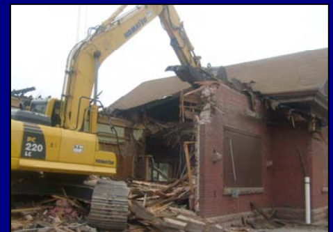
EWI performed the demolition of a depot building for a Major Railway Carrier without any track downtime.
